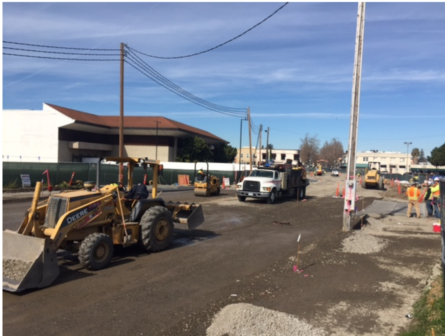
New Murphy Avenue roadway graded and placed compacted AB section. Preparing for paving.
