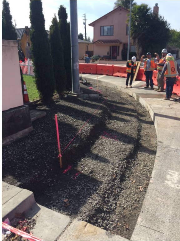
SE corner of Iowa/Murphy sawcut and graded with AB. Ready to pour back sidewalk and directional ramps.
